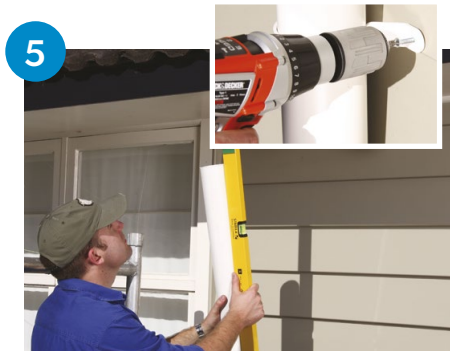
Use a level or plumb line to mark where the downpipe will sit against the wall. Ensure downpipe clips are spaced no more than 1.2 metres apart and the first clip is a maximum of 200mm below the downpipe bend. Downpipe clips to be secured with two stainless steel screws.
