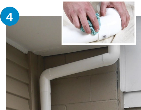
Solvent cement all remaining elbows to downpipe on ground, before completing offset installation.
